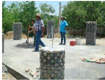
Figure 3. Circular column using reinforced plastic bottles Source: Building support columns from plastic PET bottles.
