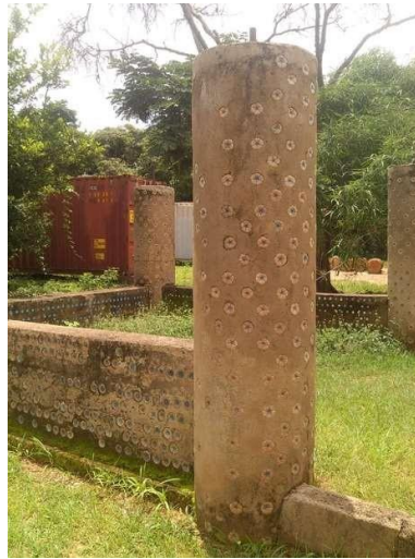
Figure 9. Column arrangement and adjoining wall made with plastic bottles, cement and steel reinforcement Source: Field study (2016).
